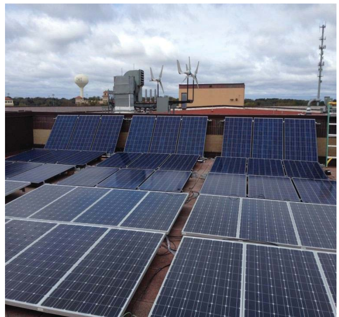
Figure 7: Solar Panels and Wind Turbines in the SMART Lab.
